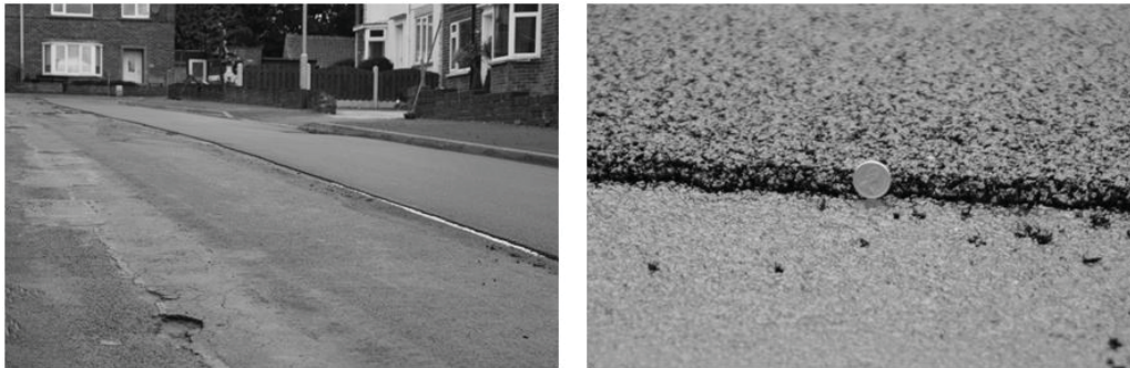
Fig. 9: Steelflow 15 mm on existing worn out road surface without the need for planning of original material.
