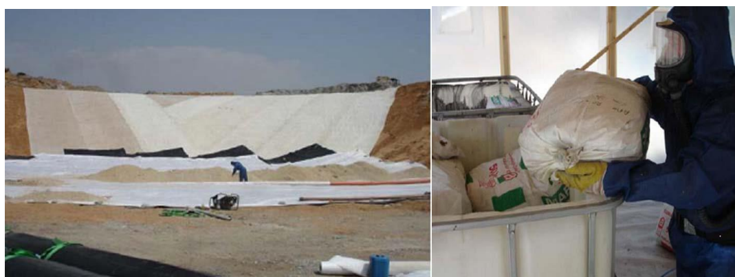
Fig. 1: View the construction of the pilot disposal site for asbestos waste (Prefecture of Kozani 2012)
